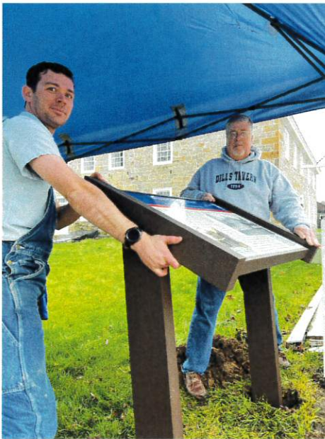
Christopher D. Brown (left), Assistant Director of Civil War Trails, Inc. and Doug Riley; CWT sign installation at Dills Tavern.
